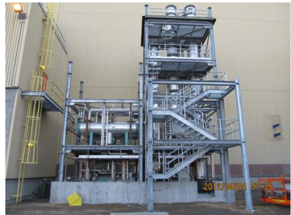
Figure 2: Methanol Purification System Modules
